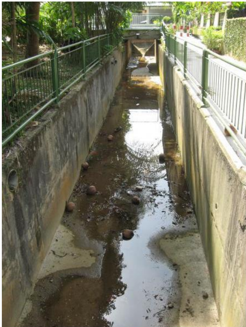
Typical stormwater drainage channel Singapore
